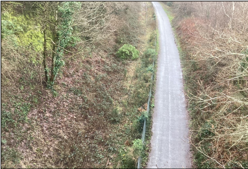
View from Tors Road Bridge on 24 th February 2024 looking west to Plymouth showing the currently overgrown track alongside the cycle way towards Meldon (Photo: Tony Hill).
