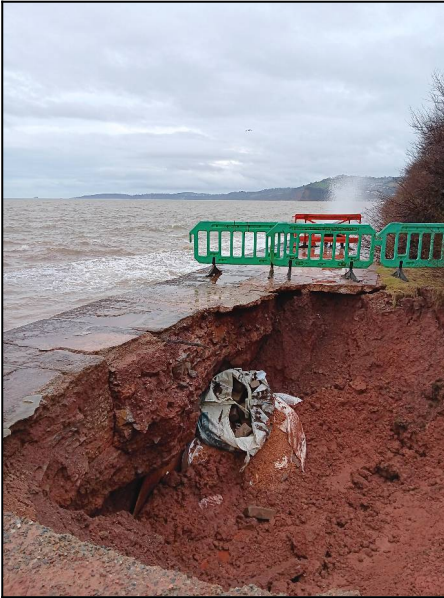
Damage to the wall at Sprey Point, Teignmouth, taken on 26 th January 2026. (photo: Sue Baxter).
